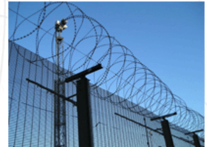
CCTV & Fence Intrusion Detection System
