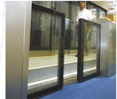
Platform Screen Doors
