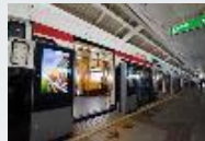
Platform Screen Door
